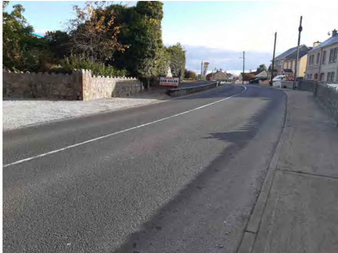
Gap in Footpath on R521
