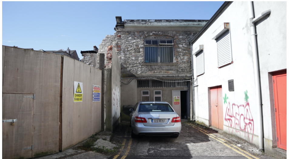
Elevation to Glenworth Lane showing stone wall to be taken down and reconstructed.
