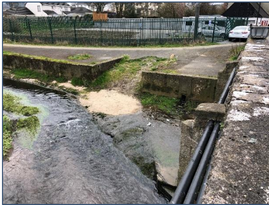
Plate 2-3 View from the Wolfetone bridge of the slipway leading to the River Loobagh (FW1) and associated asphalt and paved path behind site (BL3).
