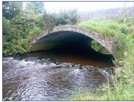
Plate 2-6 Bridge over which the R515 runs over, comprised of corrugated metal (BL3) with the overgrown ornamental flower bed (BC4) visible atop the bridge. The line of rocks running across the Loobagh is also visible.
