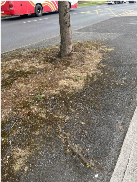
Tree No.1691 roots lifting the surrounding tarmac path next to Circle K Roxboro.
