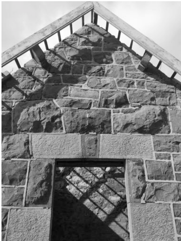
Cementitious pointing to be removed
