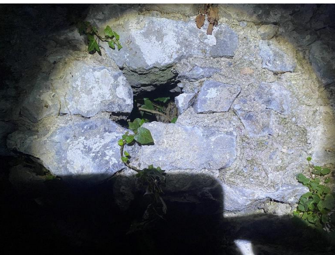
Plate 9 One of the many crevices in the stone walls at the proposed development site.
