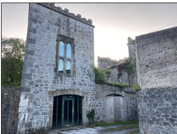
Plate 2 Eastern side of the proposed development building. The structure to the rear is where the roof has collapsed.
