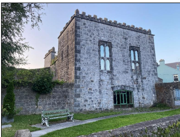
Plate 3 Southern façade of the building. The stonework here was in good condition and well sealed.
