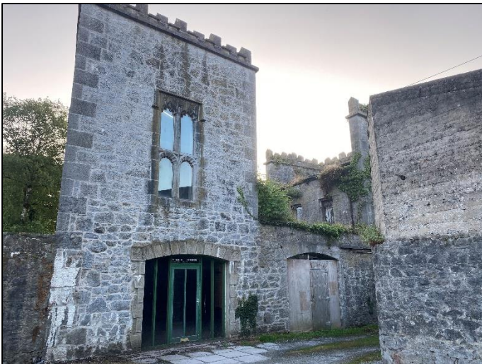
Plate 2 Eastern side of the proposed development building. The structure to the rear is where the roof has collapsed.
