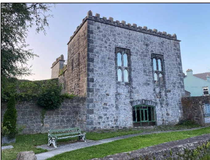
Plate 3 Southern façade of the building. The stonework here was in good condition and well sealed.
