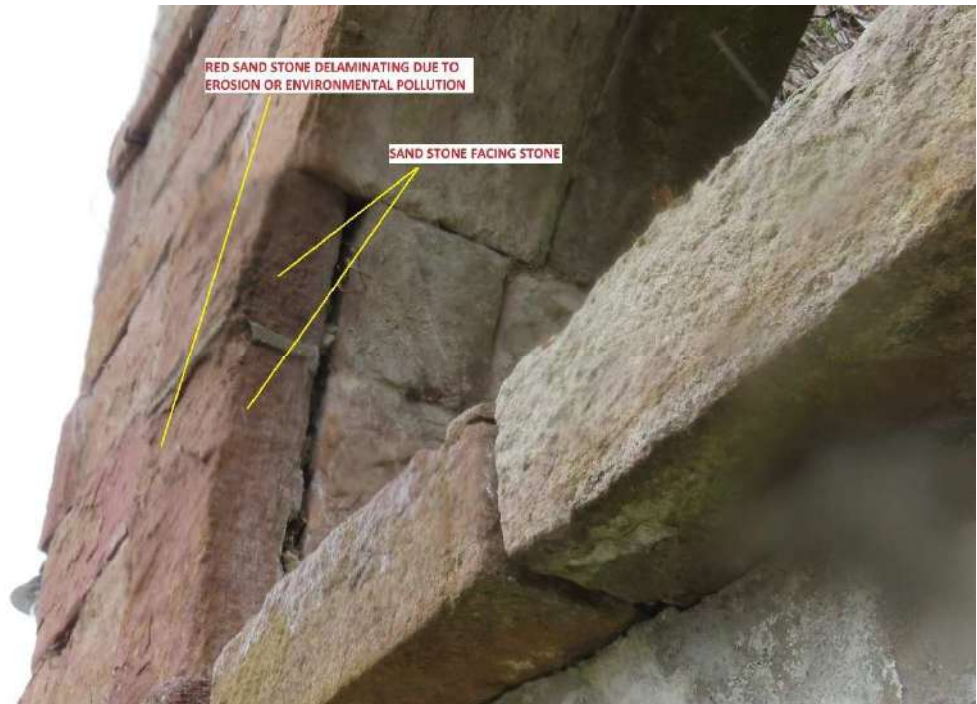
Photograph 016. Showing facing stones & sandstone delaminating (environmental pollution?)
