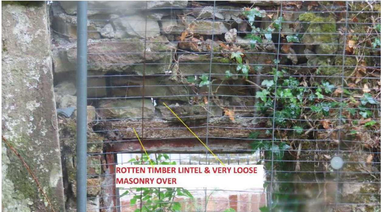
Photograph 021. Showing rotten timber lintel & very loose masonry over on the South-West gable wall.
