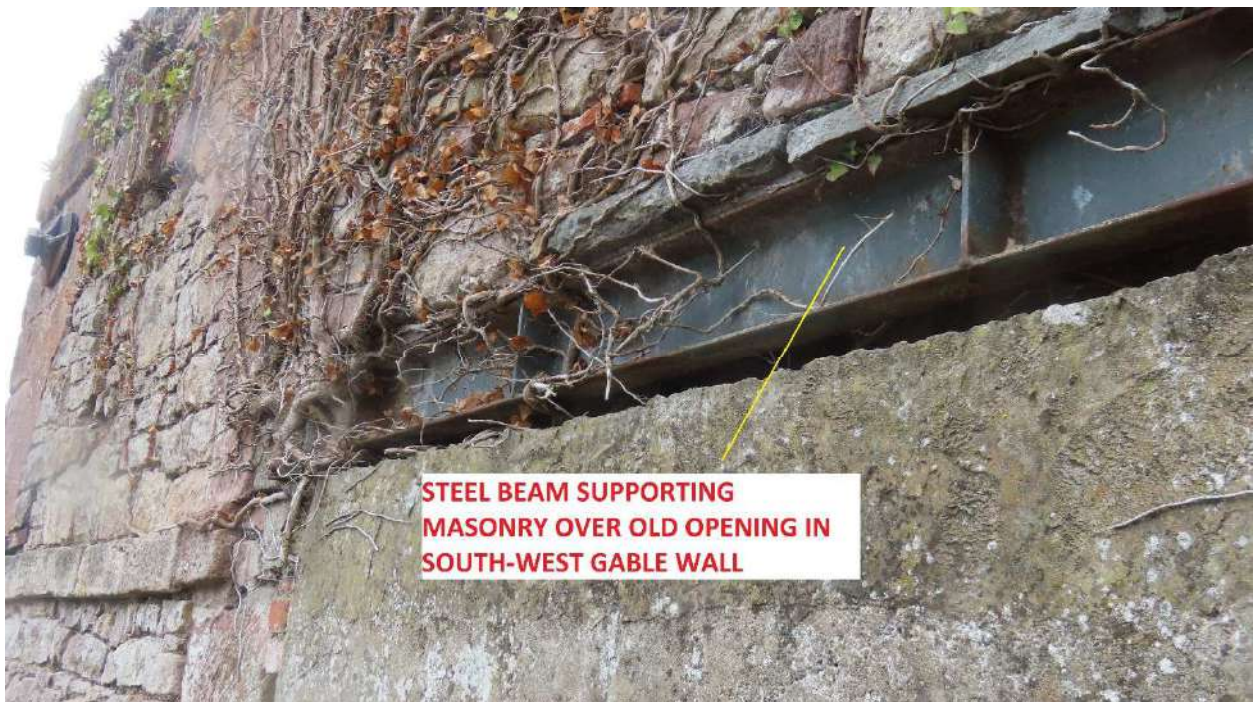
Photograph 017. Showing steel beam over old door opening on the South-West gable wall with concrete infill under & masonry infill to the original stone arch.
