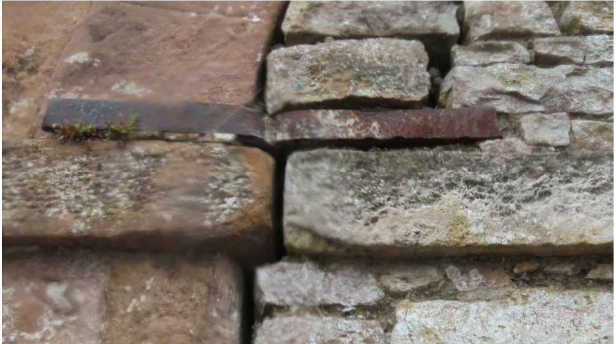
Photograph 020. Showing steel anchor for the tie bar in the South-West gable at the spring of the arch.
