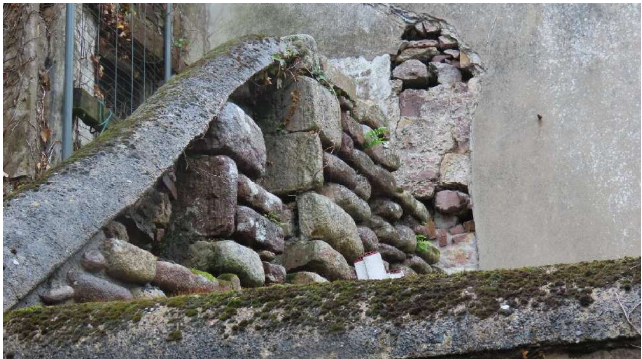
Photograph 022. Showing poor structural condition of stone steps handrail wall which is over the adjoining property backyard.
