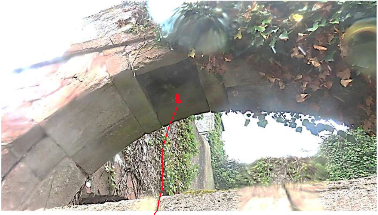
Photograph 010. Inset sand-stone missing near crown of arch, facing stone in position back & front are in place.
