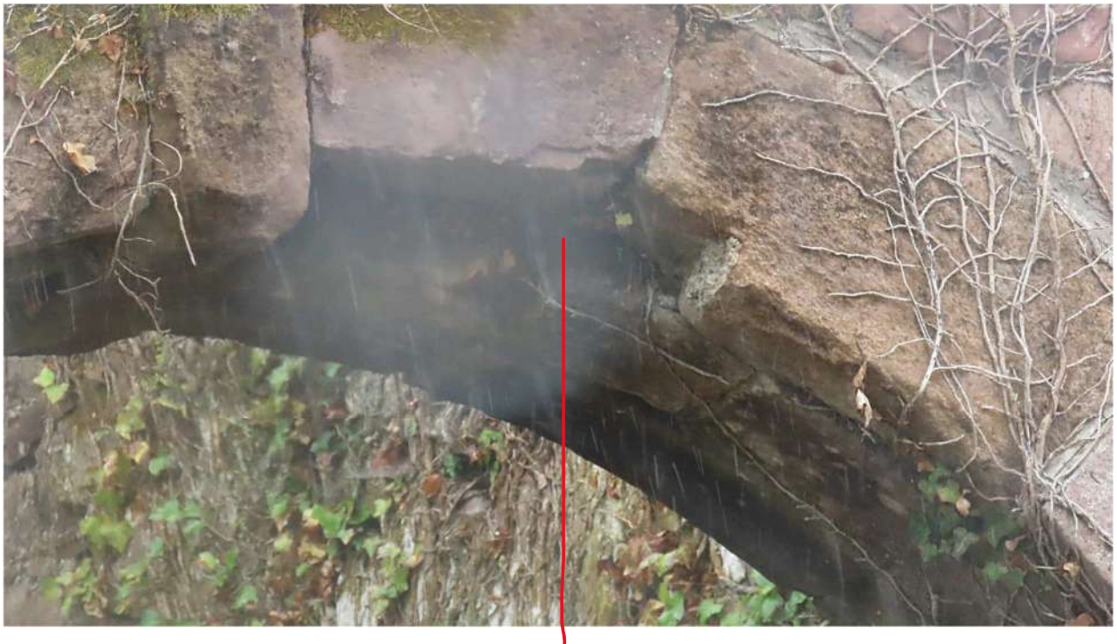
Photograph 011. Inset sand-stone missing near crown of arch, and one facing stone is broken with a missing section.
