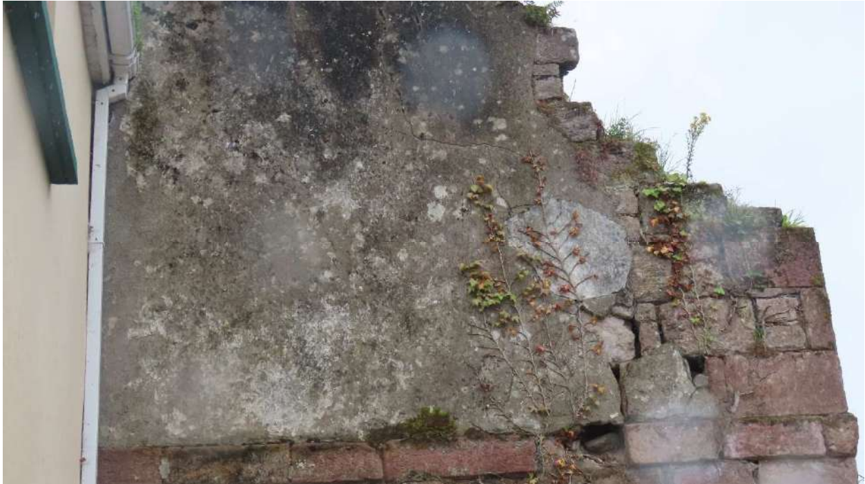
Photograph 018. Showing loose & cracked plaster on the North-East Gable.
