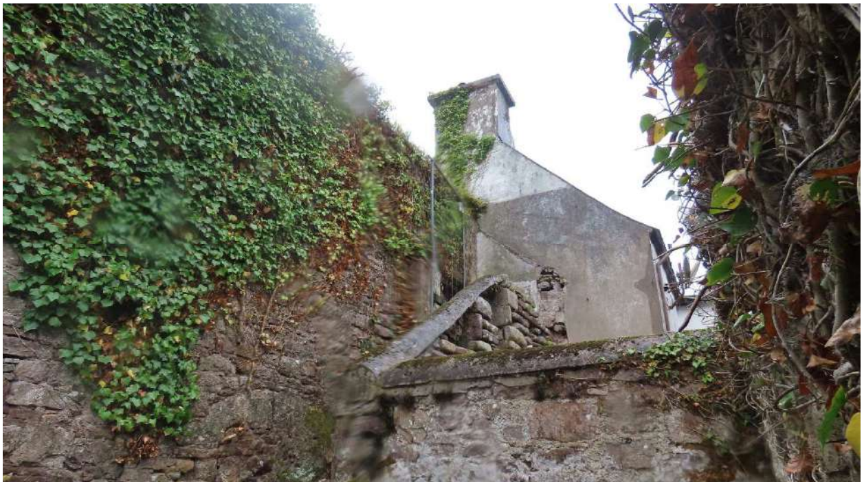
Photograph 009. Back wall & stone steps hand-rail wall (in very poor condition) at the South-East face.
