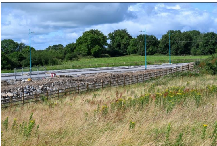
Plate 12 Road and associated infrastructure under construction on the southern boundary of the site (Planning Reference 19/8011). This development has already fragmented the site.
