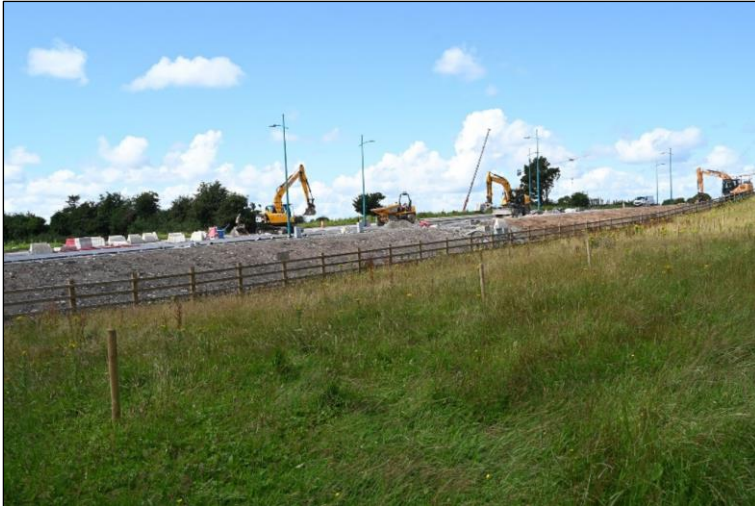
Plate 13 Road and associated infrastructure under construction on the southern boundary of the site (Planning Reference 19/8011).
