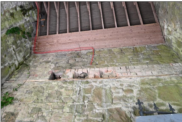
Plate 29 Ledge previously used by the Owls with new wiring installed. There is some whitewash on the walls, but this could be from a previous nesting season.
