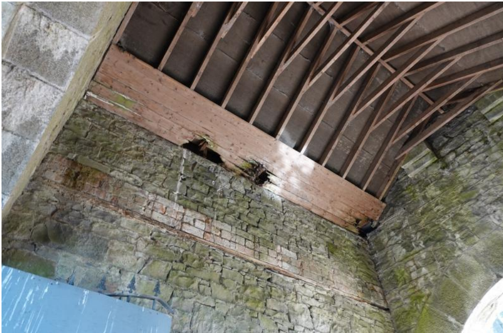
Photograph 3: Whitewash and rotten timbers under the stone archway.
