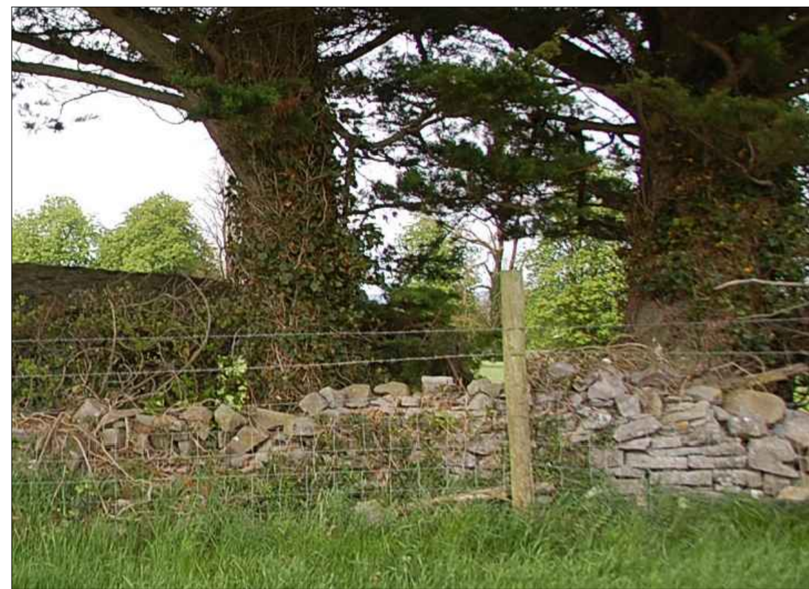
7 PHOTOGRAPH TYPE 4 - EXISTING SOD AND STONE WALL TO BE REPAIRED
