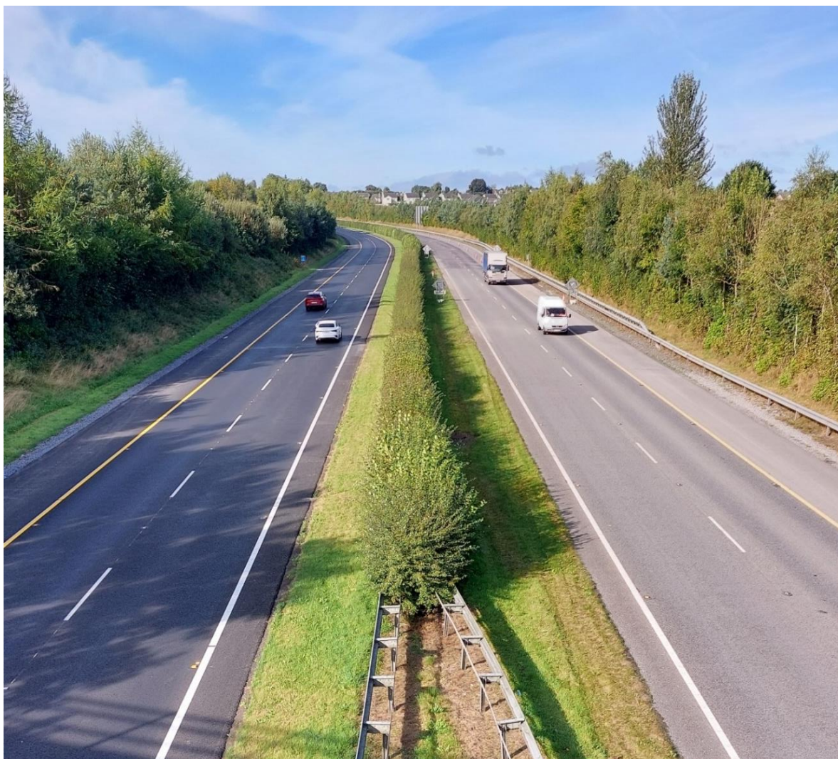
Figure 3.5. Resurfacing of the M7 motorway near Castletroy (between Junctions 28 and 29) with the southbound carriageway (left) complete in the photograph.
