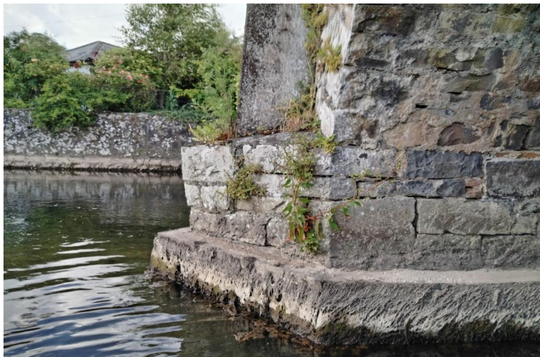
Figure 4. Damaged cutwater on the downstream side.
