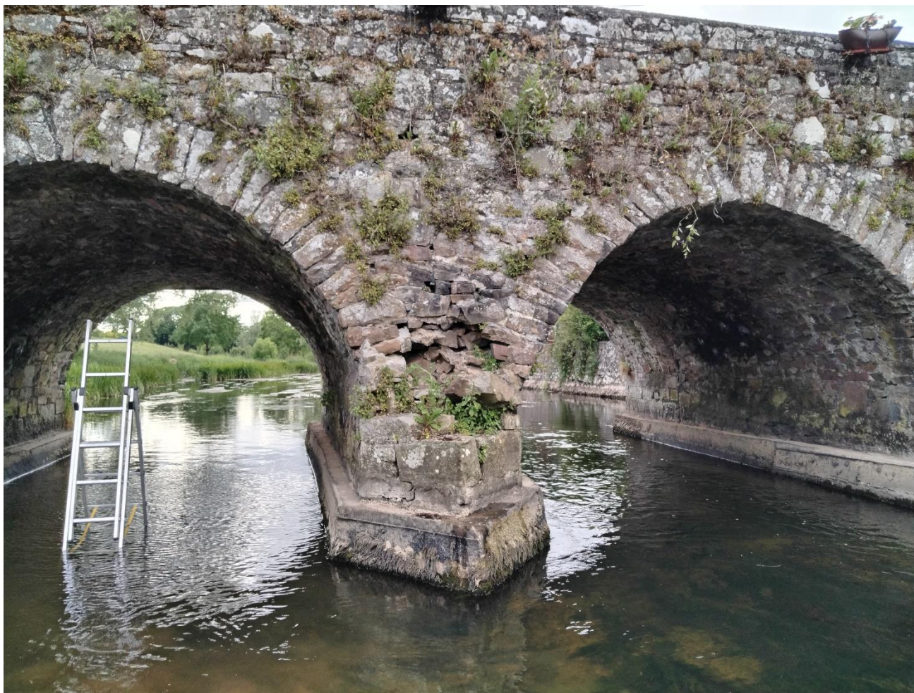
Figure 3. Damaged cutwaters on the upstream side.
