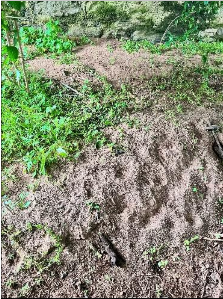
Image 2-2 – Unidentifiable prints under arch 4 of bridge
