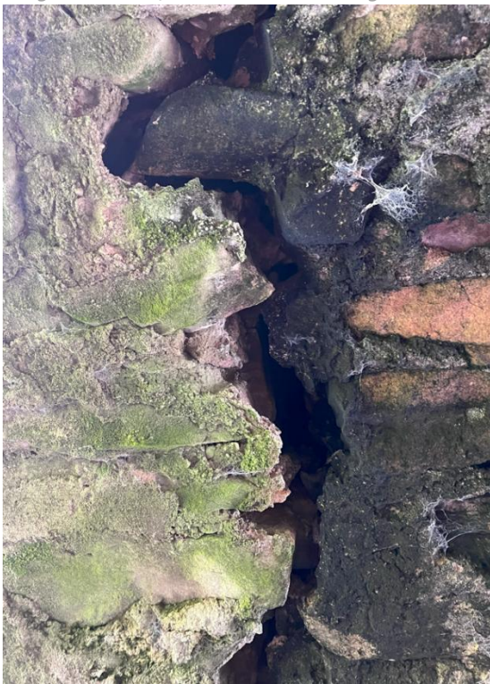
Image 3-3. A large crack present on the underside of one of the arches.
