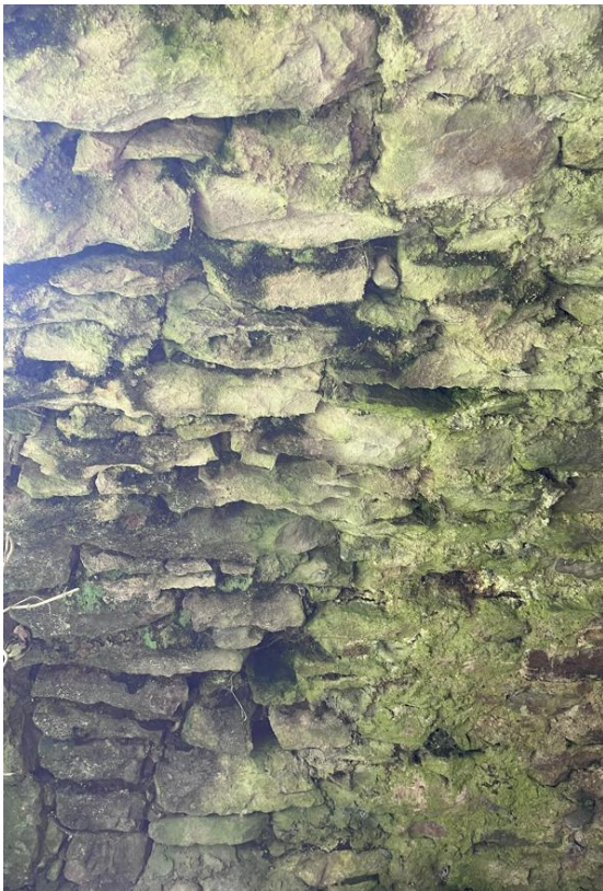
Image 3-4. Cracks, holes and dislodged mortar on the underside of one of the arches.
