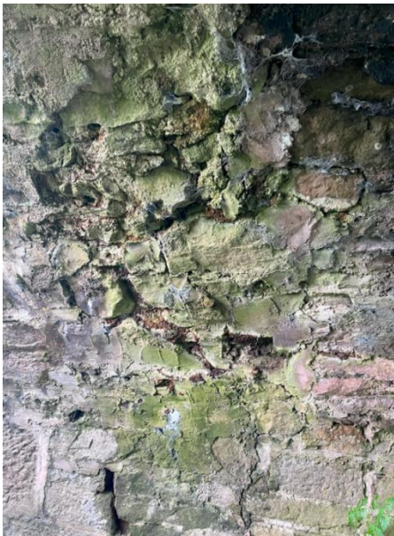
Image 3-2. Cracks, holes and deteriorating stone and mortar on the underside of one of the arches.
