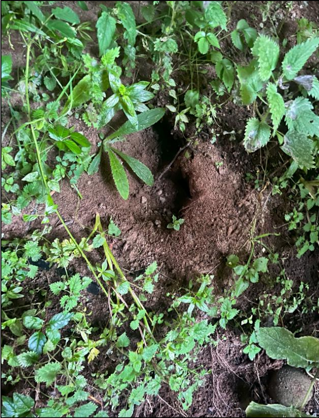
Image 2-3 – Arch 4 – Survey 2, south arch of bridge, light digging/rooting
