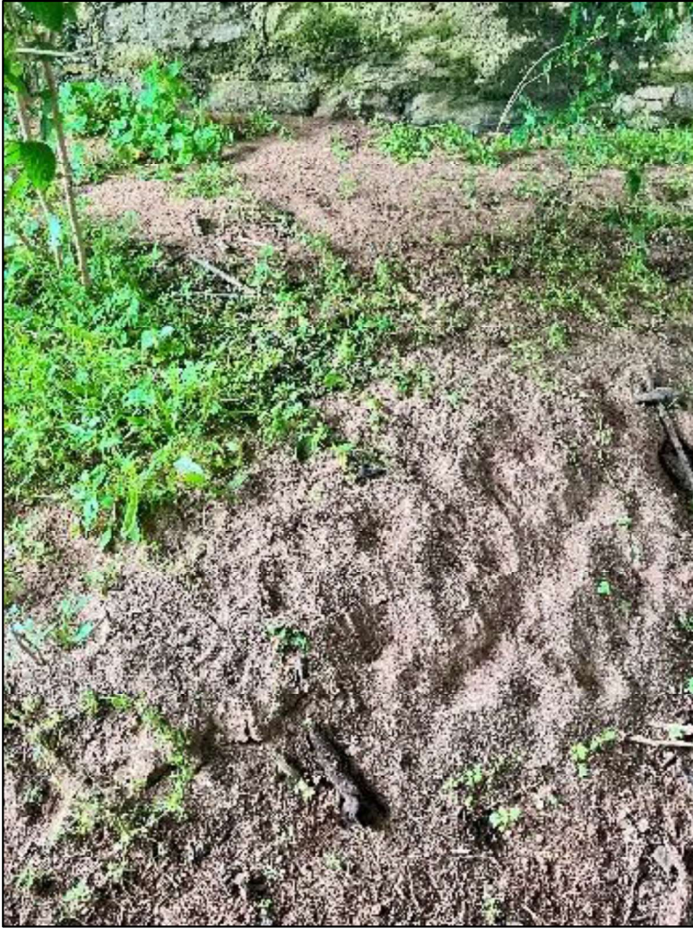
Image 2-2 – Unidentifiable prints under arch 4 of bridge
