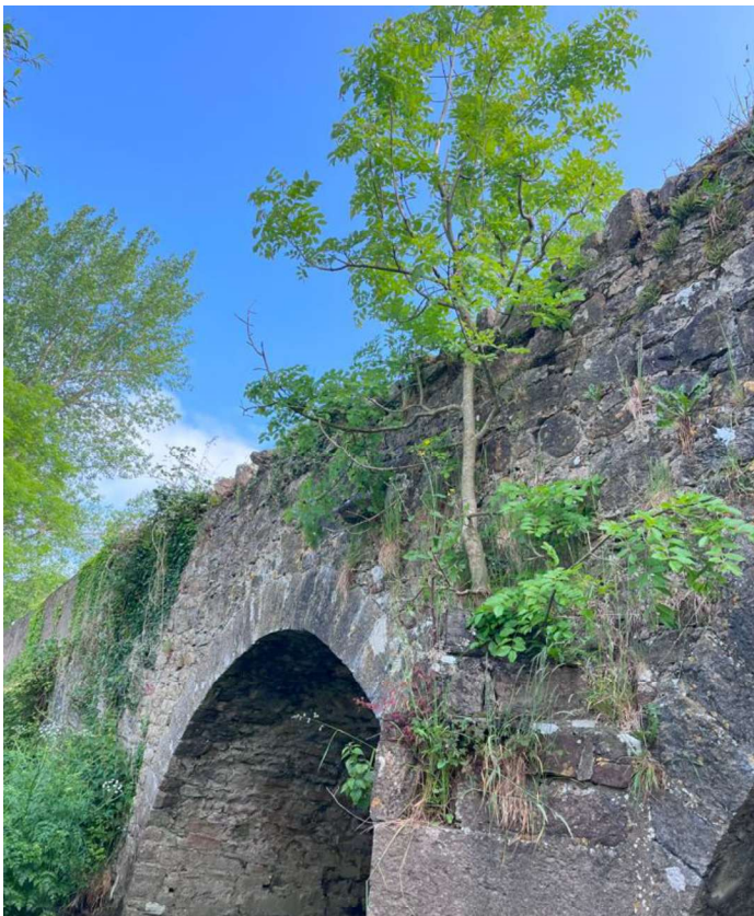
Image 3-5. Vegetation present on the upstream bridge abutment and cutwater.
