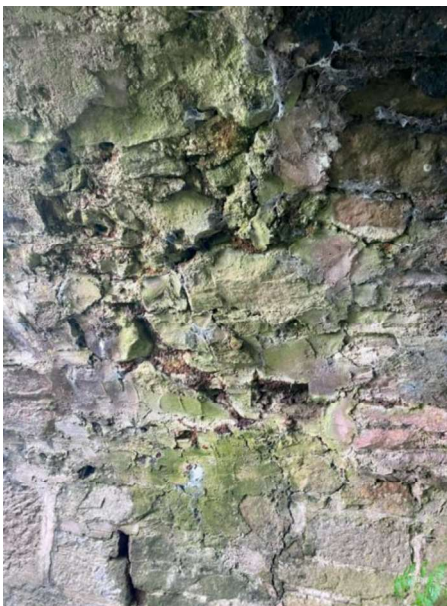
Image 3-2. Cracks, holes and deteriorating stone and mortar on the underside of one of the arches.
