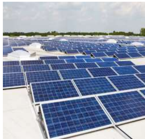
Figure 5: Solar Photovoltaic Panels
