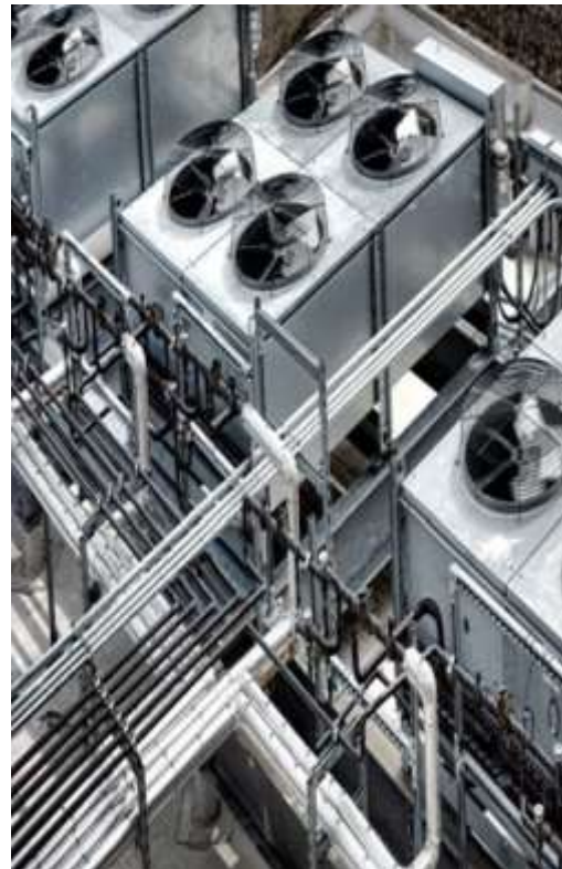
Figure 7: Outdoor Condenser Unit
