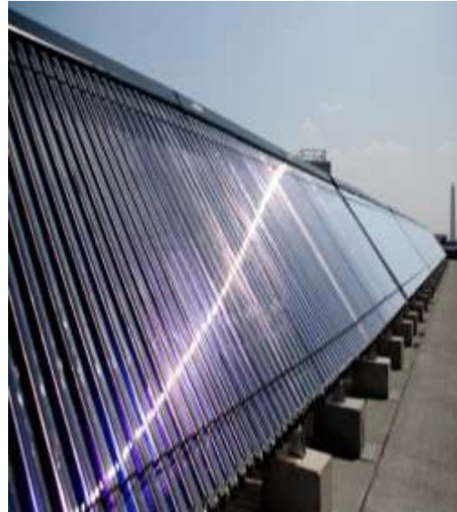
Figure 6: Solar Water Heating Panels
