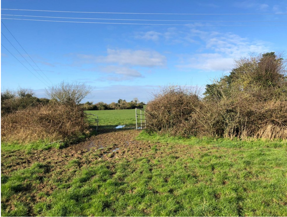
Image 1: Photograph taken on the proposed development site. Ponding observed on site after prolonged period of rainfall.
