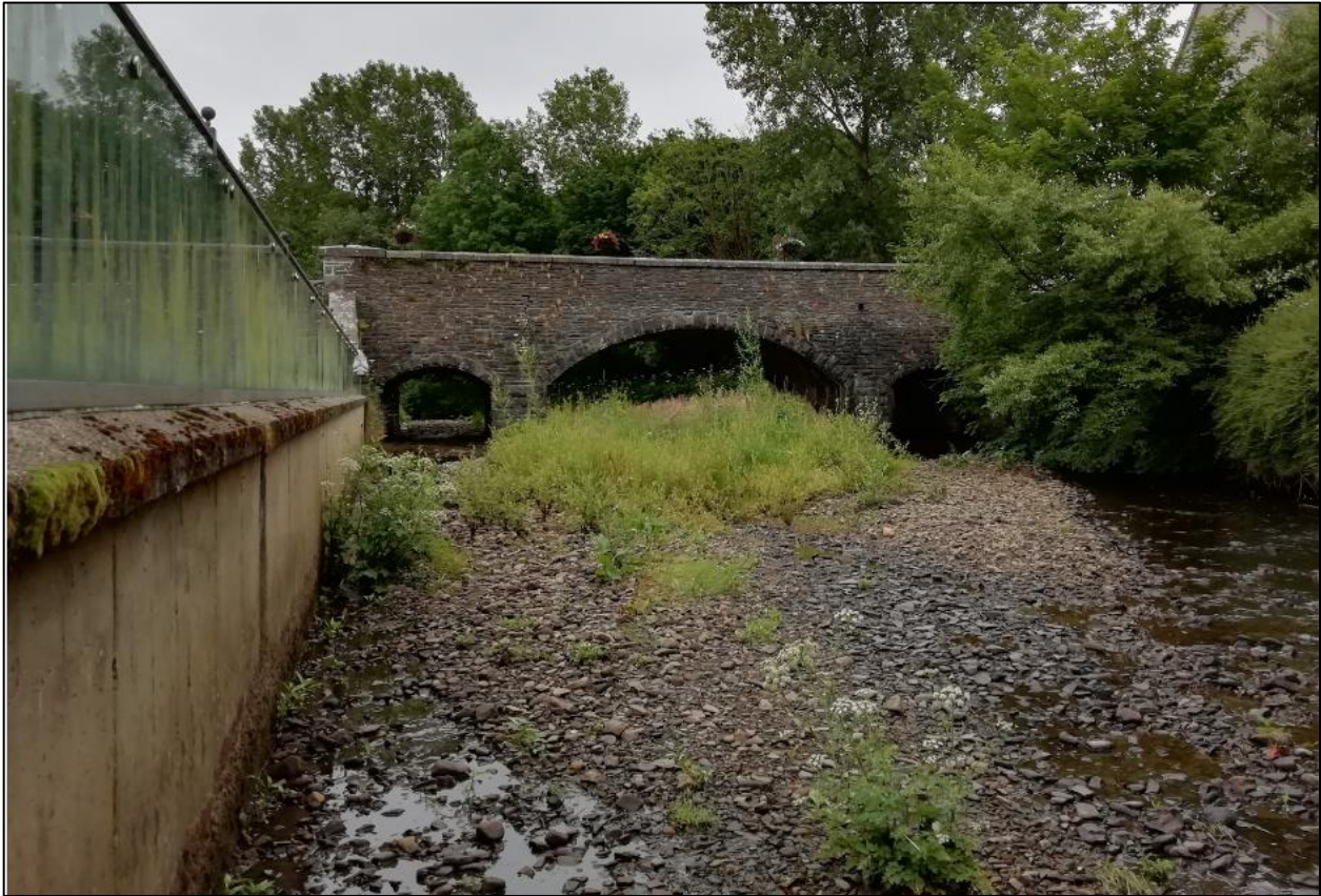
Figure 1-2: Gravel deposit downstream of Athea Bridge (Taken on 18/06/20)
