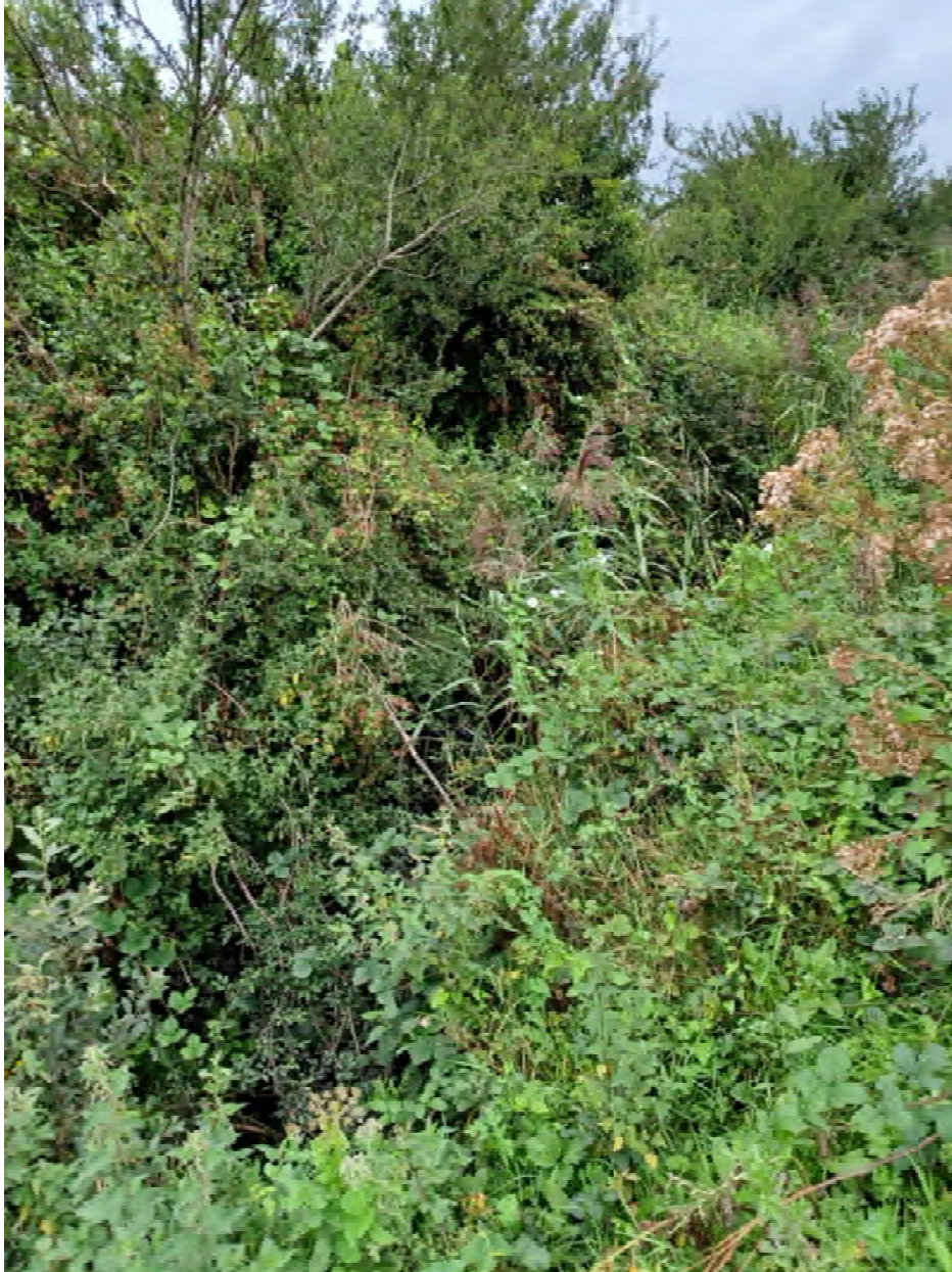
Image 6: Overgrown nature of OPW channel
