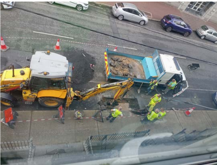
August 2022 – Same Irish Water pipe bursts. Further works required.
