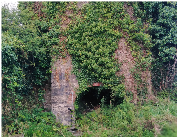
Existing historic limestone structure to be restored and setting enhanced with sympathetic paving scheme
