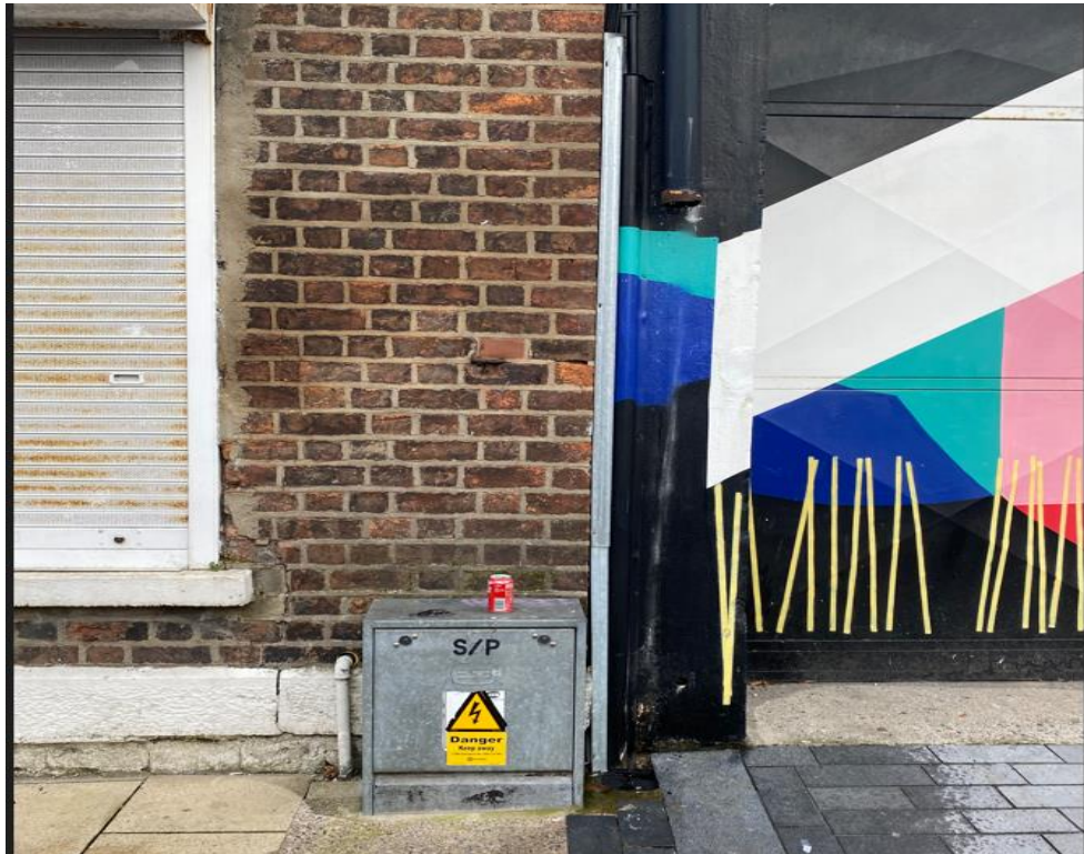
Figure 7 – Existing ESB Mini pillar between 33/34 Thomas Street
