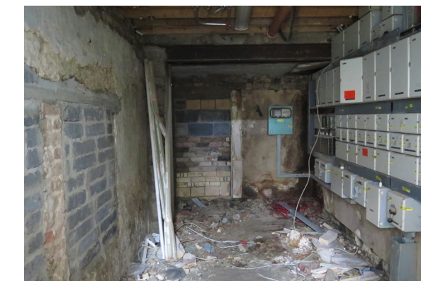
Photo 31: M&E Fuse & Switchboards in Basement Return
