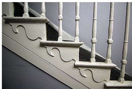
Photo 13: Thread ends to Stairs and Original Balusters
