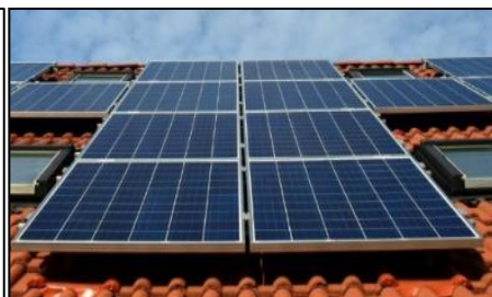
Figure 2 – Typical Solar PV panels
