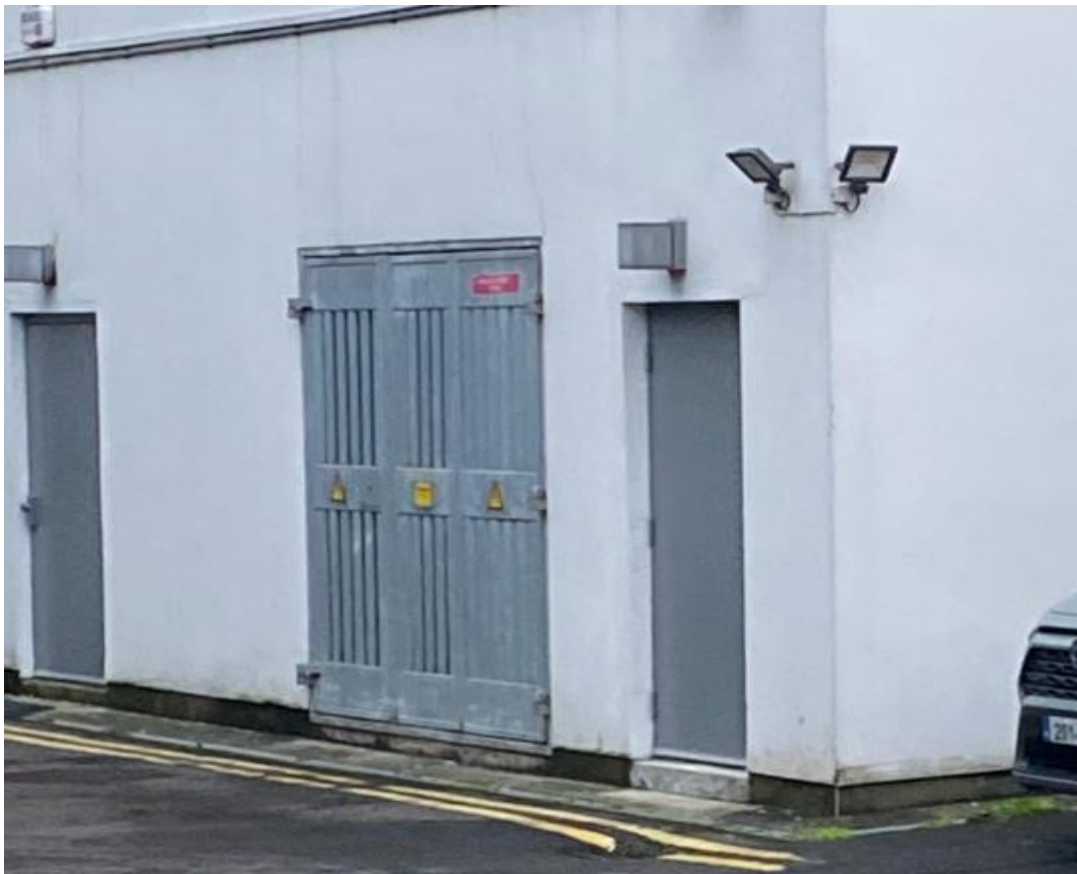
Figure 6 – Existing ESB Substation at 59/60 O'Connell Street
