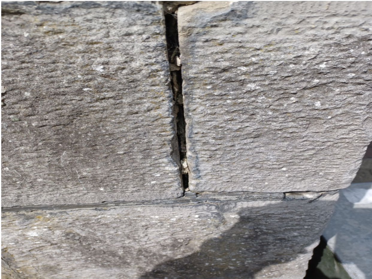
Figure 8: though located on Nicholas Street, the dimensions and depths of the cracks in this stone work, close to where a sign is to be erected is typical of those found in such structures throughout the area. No traces of bats or birds were found in any.
