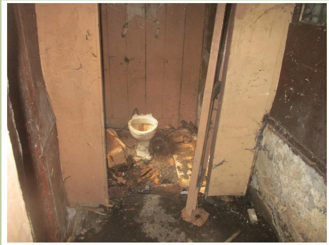
Toilet cistern in the ground floor W/C
