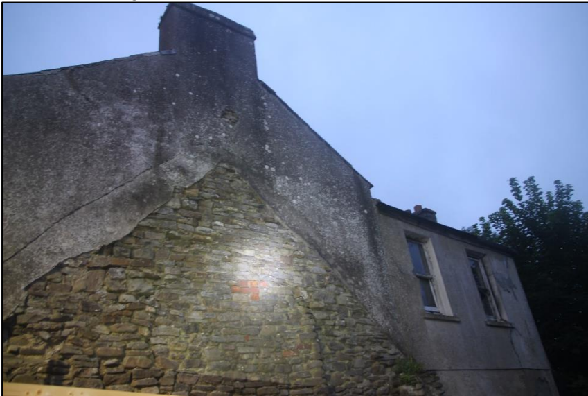
Plate 3 Building for demolition, side of site. Bat Roost Potential 'Low'. No bat emergence.
