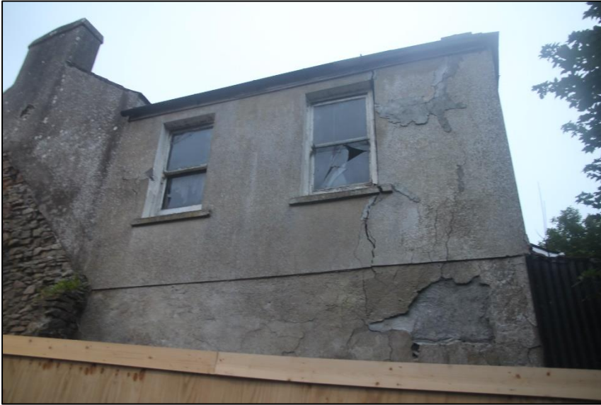
Plate 2 Building for demolition, side of site. Bat Roost Potential 'Low'. No bat emergence.
