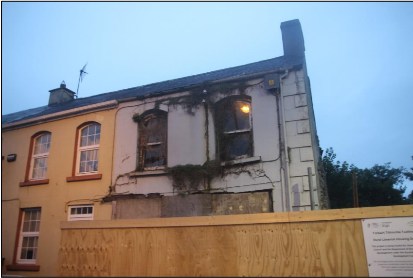
Plate 1 Building for demolition, front of site. Bat Roost Potential 'Low'. No bat emergence.
