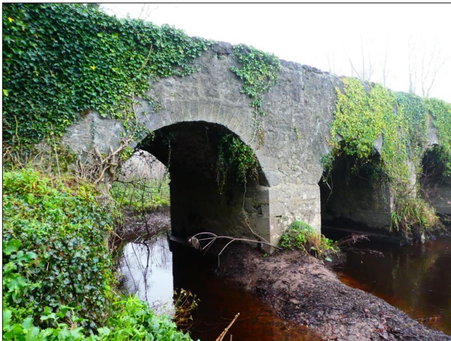
Plate 8 This site was also visited during winter 2020 and Ivy growth was noted on the bridge structure, which was not present at the time of the visit in March 2021. It is unclear when this was removed.
