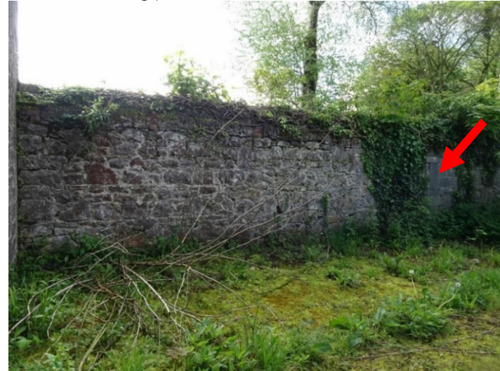
South garden wall This wall is contemporary with the building. The arrow indicates the location of the mason's mark.
