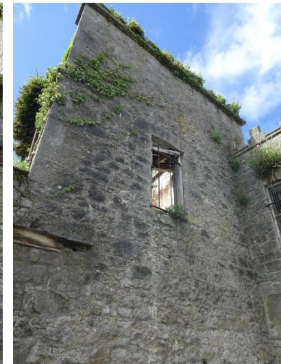
7. First floor window_north building (derelict)
