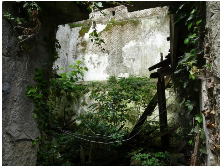
26. First floor collapsed
