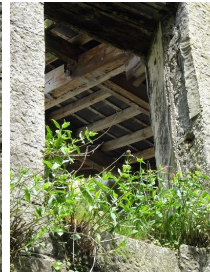
27. Part of roof extant_rest fallen into building
