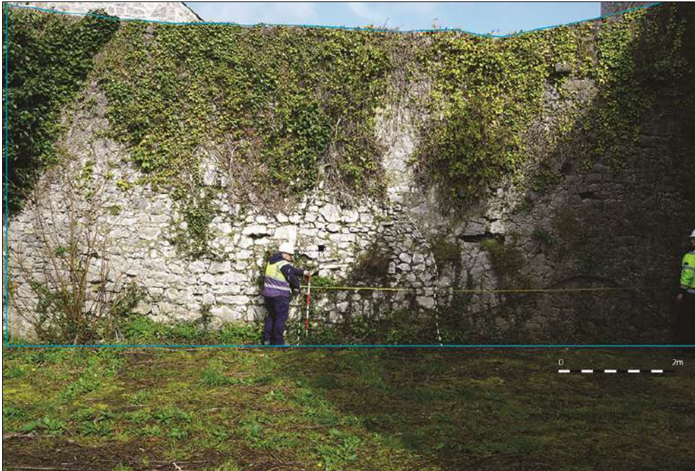
Plate 4. The south face of the boundary wall as seen from Fuller's Folly. The dashed line indicates the presence of the former hole in the wall which allowed access to the yards at north (photo by writer).
