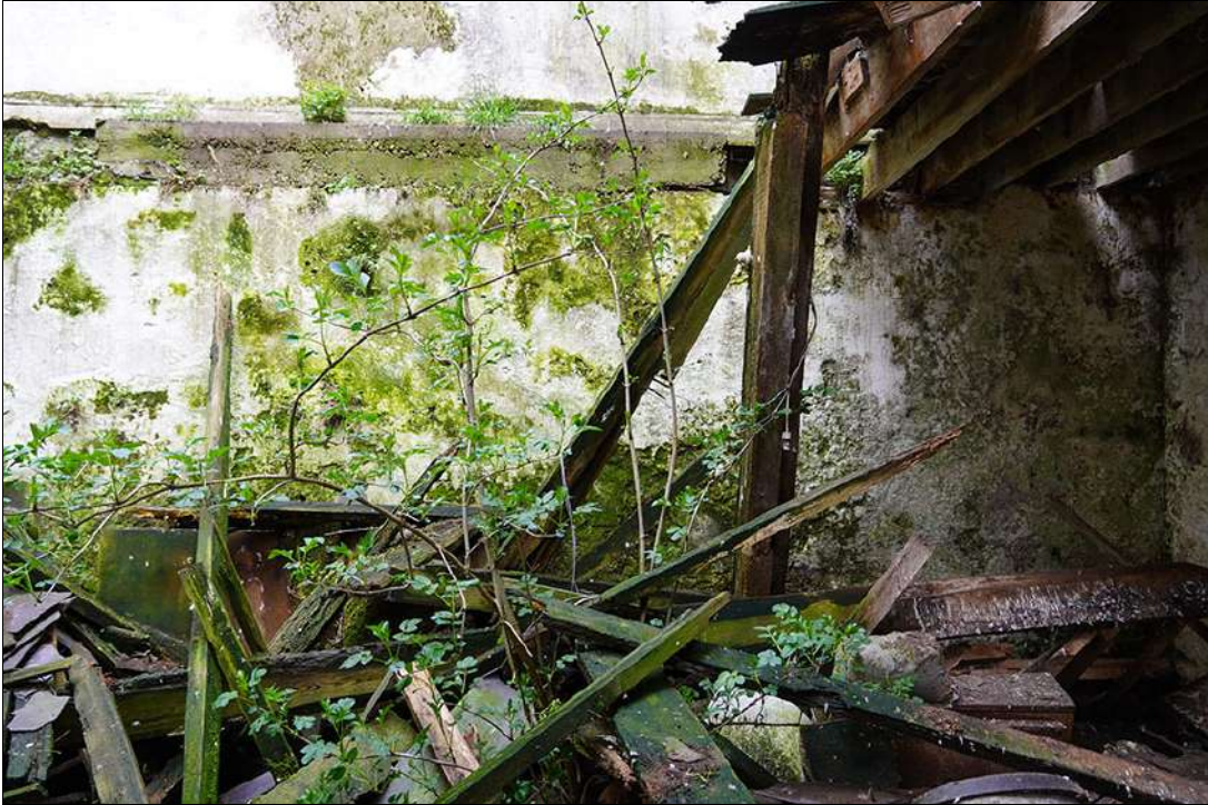
Plate 3. Debris from collapse and assorted items of possible cultural heritage interest in the northern building, from S.
