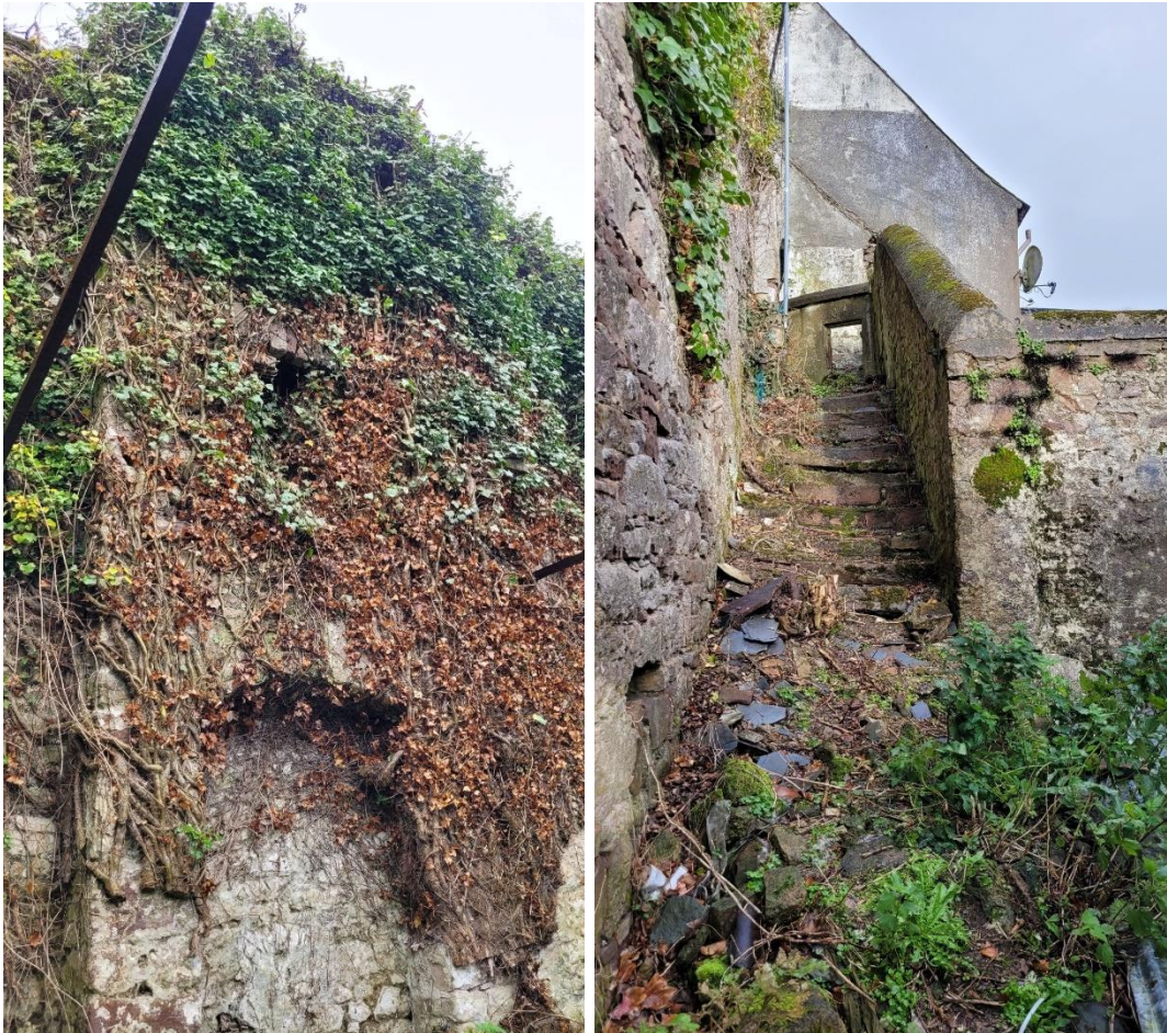
Image 4-3: Ivy covered internal wall and stone steps to the rear of the building.
