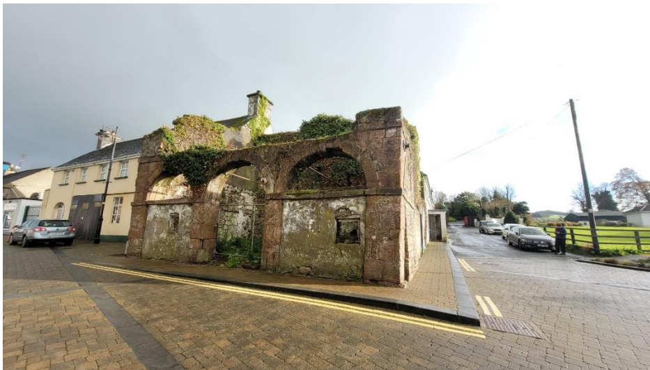
Image 3-1: View of derelict building from the front
