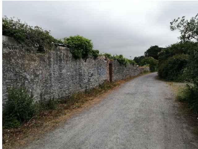
D1: South Boundary Wall
