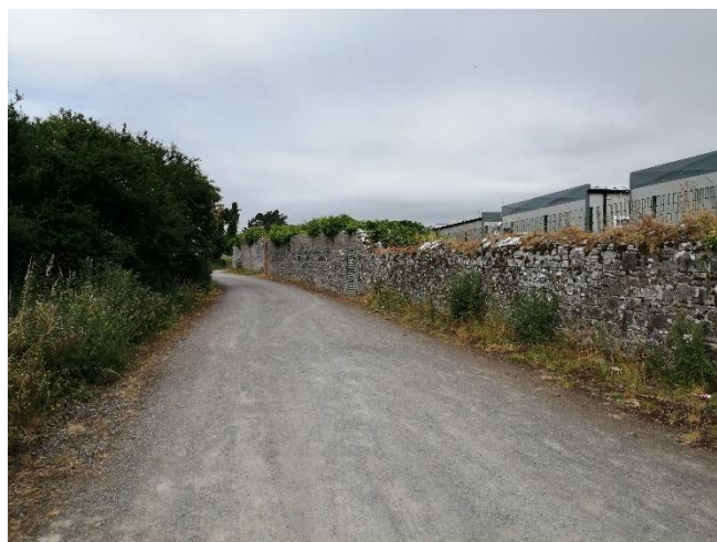
D3: South Boundary Wall
