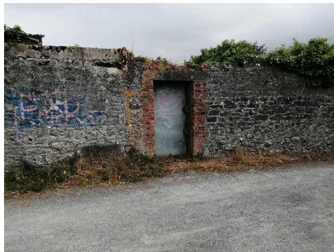
D2: South Boundary Wall
