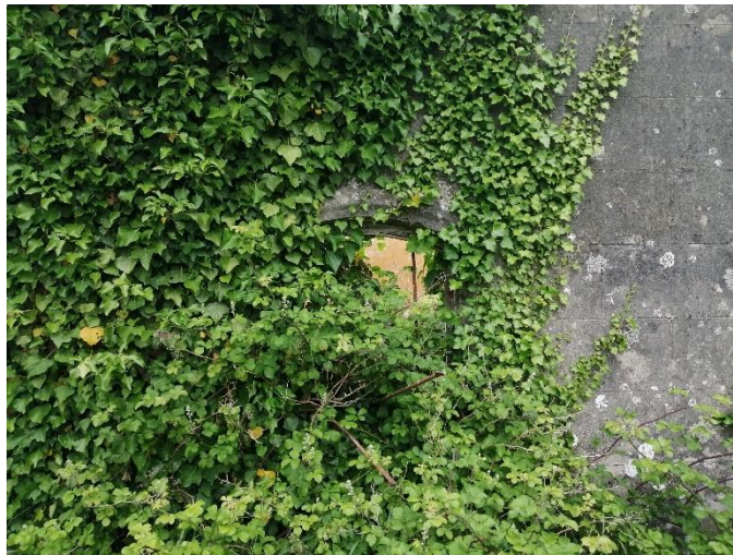
C5: Observatory South Facing Elevation, Indicating Window completely overgrown with vegetation
