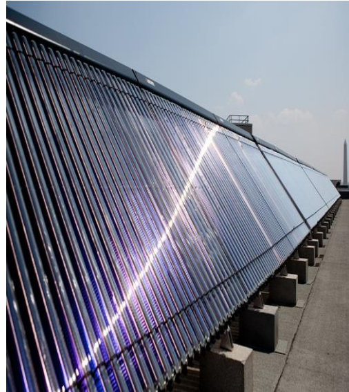
Figure 6: Solar Water Heating Panels
