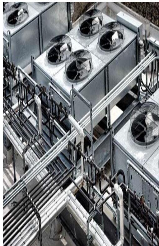
Figure 7: Outdoor Condenser Unit
