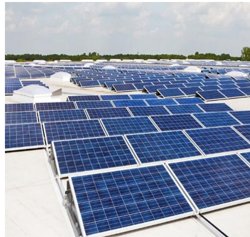
Figure 5: Solar Photovoltaic Panels
