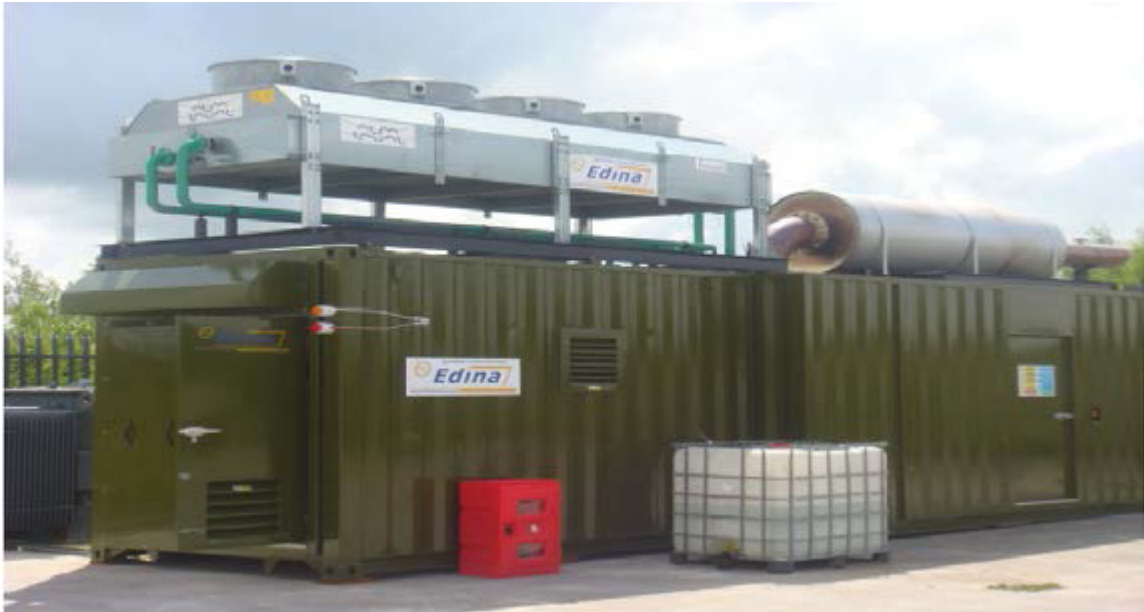
Figure 4 – Combined heat and power unit of the type in operation at Gortadroma
